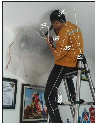
Gambar 5 Cleaning Indoor AC
